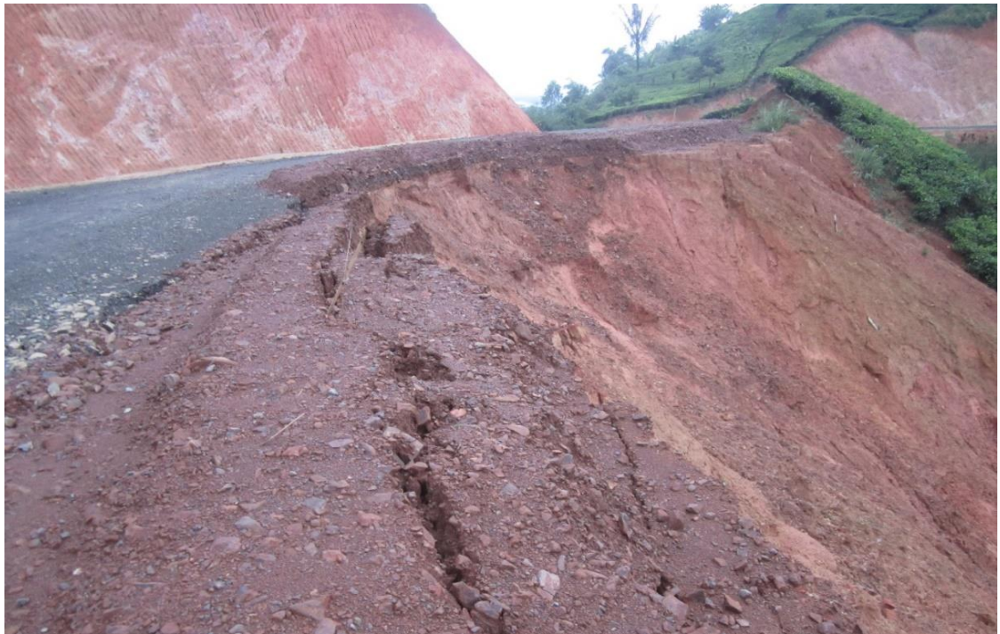
Photo 119. Landslides of soil materials on roads that have been built, Talegong District, landslide threat in the rainy season.
