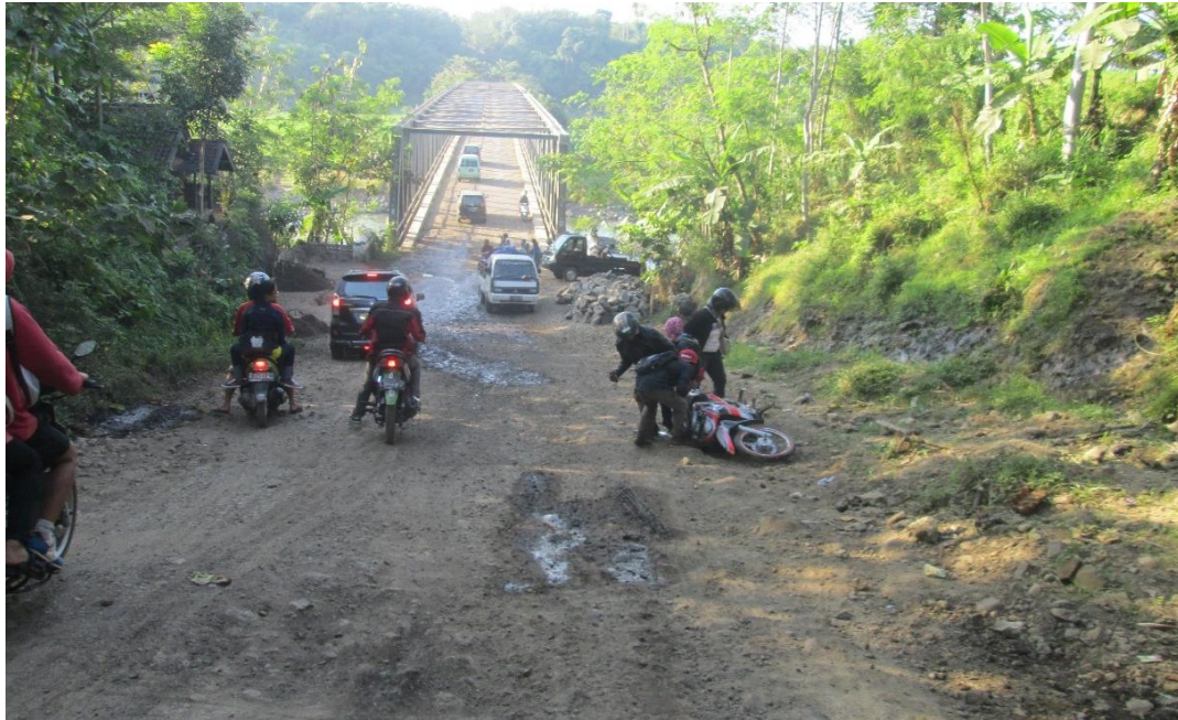
Photo 114. Before repairs were carried out, accidents often occurred on the horizontal Trans SWJ Road, the corridor of Palabuanratu-Tegalbuleud-Sindangbarang-Rancabuaya-Cipatujah-Pangandaran, Mekarmukti Distrik (South Garut).
