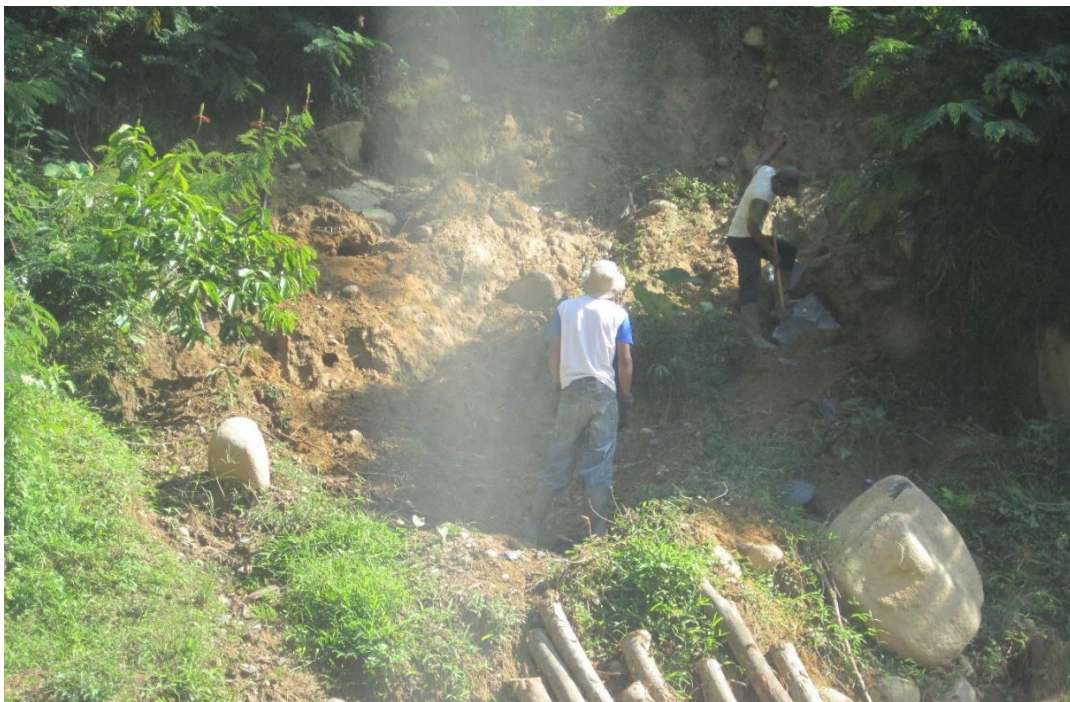
Photo 123. Local people dig stone materials as building materials from cliffs by the roadside which can cause landslides, Talegong District.
