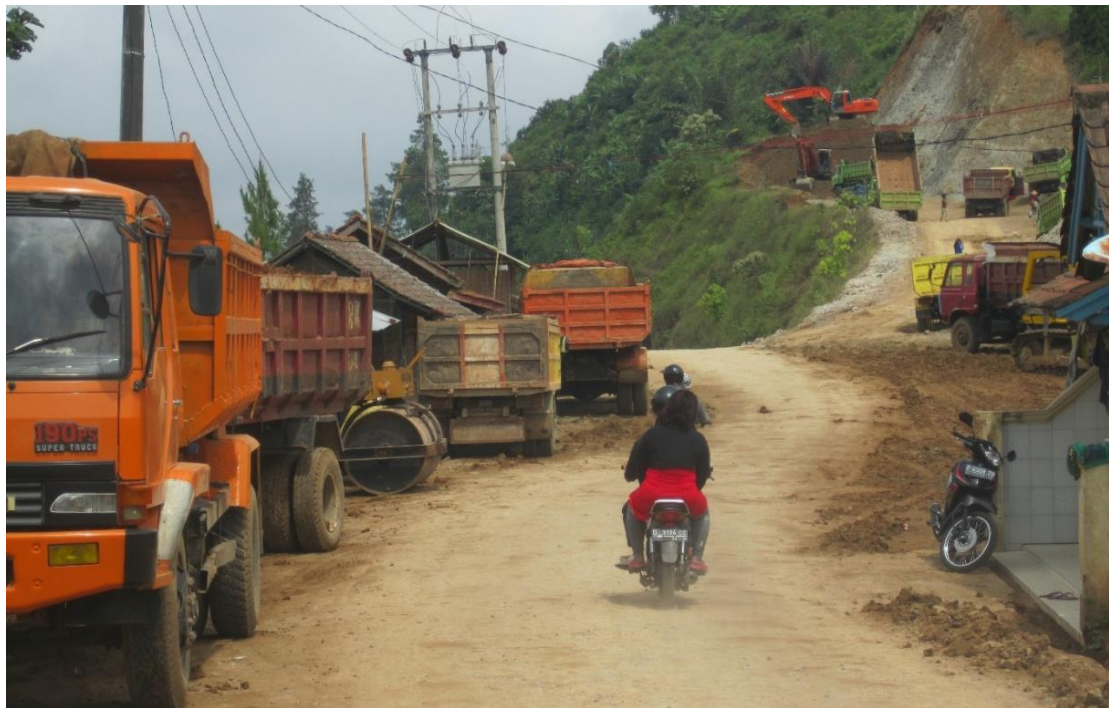
Photo 101. In the construction process of the Bandung-Pangalengan-Talegong-Cisewu-Rancabuaya Corridor Vertical Road, heavy equipment is on a steep cliff.
