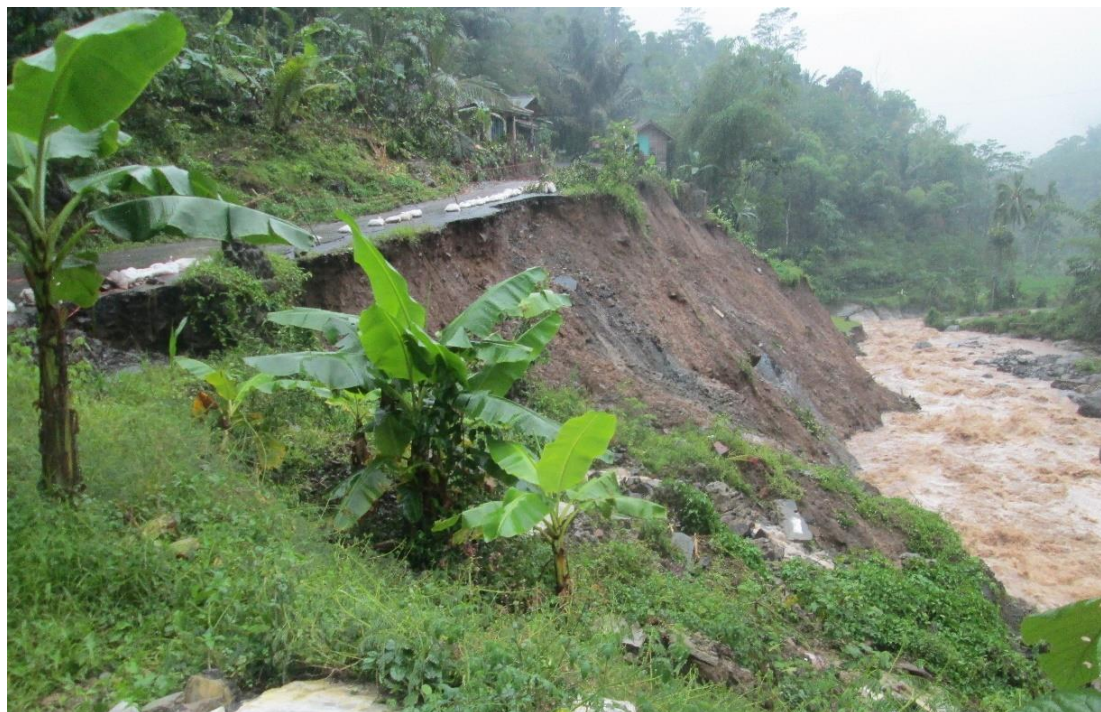
Photo 121. The road that has been finished has been eroded by the river, Cisewu District, landslide threat in the rainy season.
