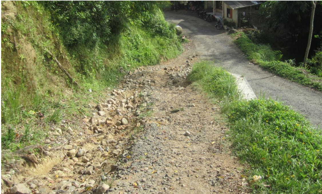
Photo 84. Puncak Hamerang-Tiwugenteng-Amlong three-way junction is very damaged and unfit.
