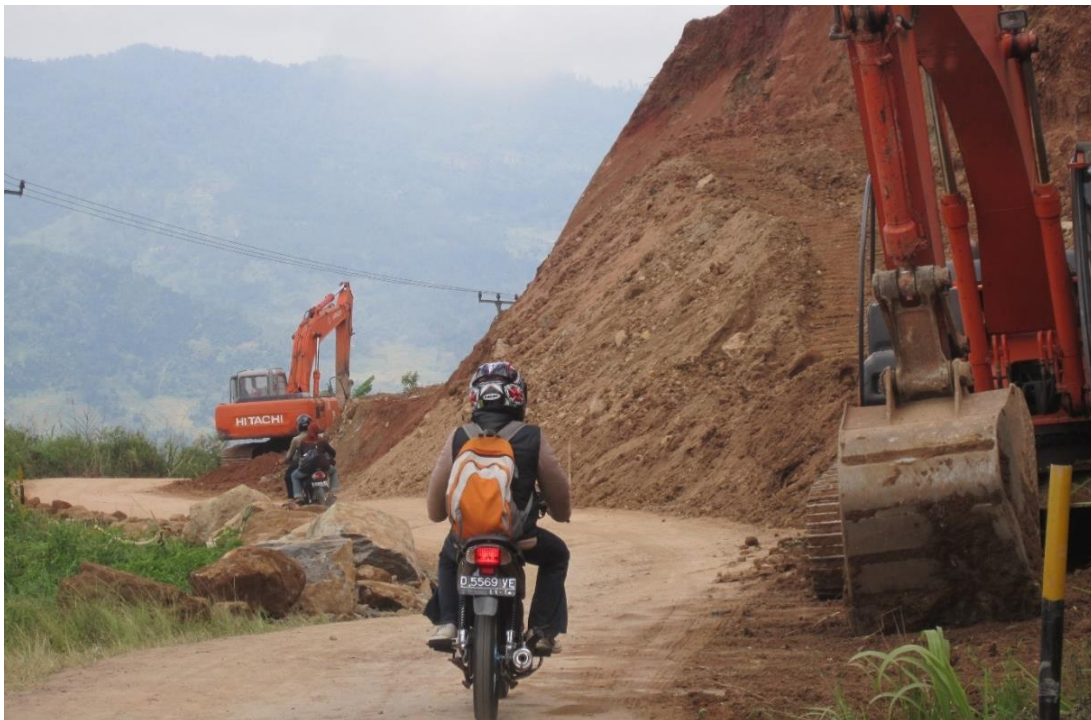
Photo 99. The Construction Process of the Bandung-Pangalengan-Talegong-Cisewu-Rancabuaya Corridor Vertical Road, is dominated by red clay.
