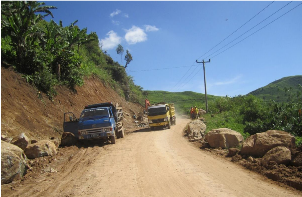
Photo 102. In the construction process of the Bandung-Pangalengan-Talegong-Cisewu-Rancabuaya Corridor Vertical Road, dismantle the boulder.
