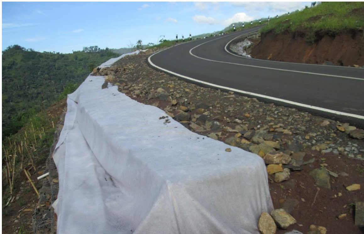
Photo 117. The threat of landslides on roads that have been built, Talegong District.
