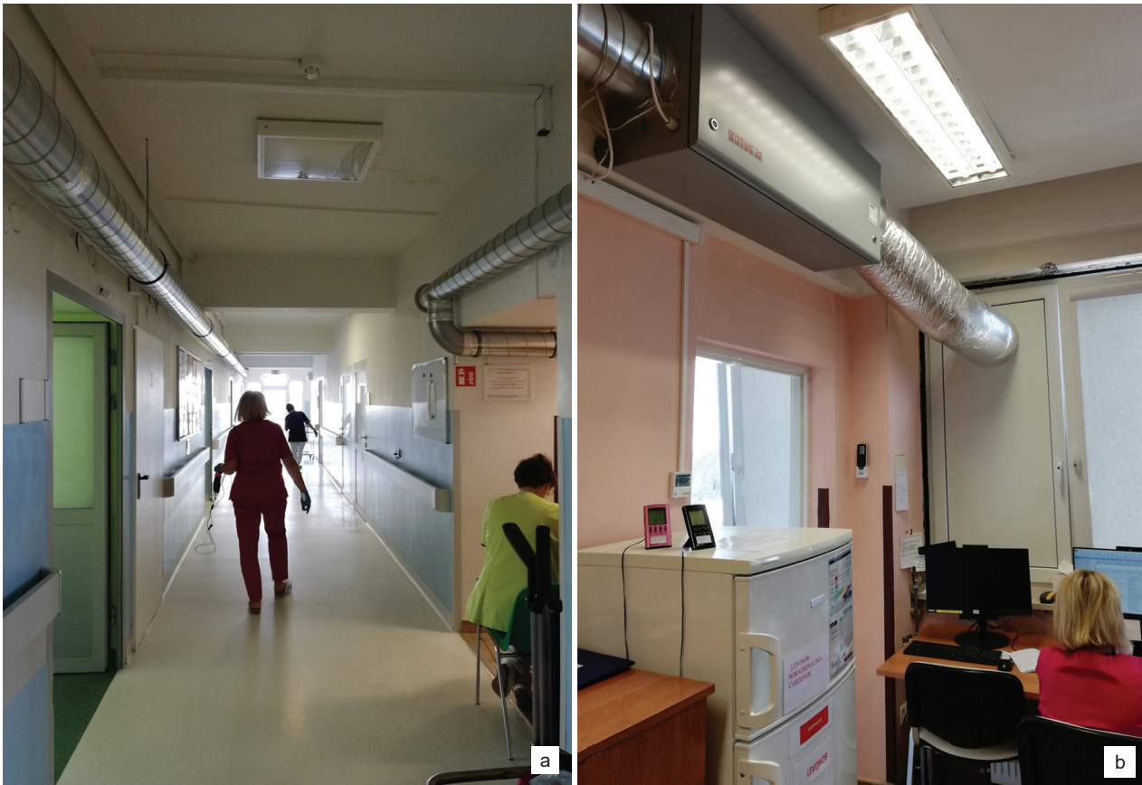
Fig. 2. Hospital in Puławy: a) corridor with visible ducts of mechanical ventilation, b) nurses' station with visible ducts of mechanical ventilation and air-conditioning – limiting ergonomics within the ward (photo by R. Strojny)
