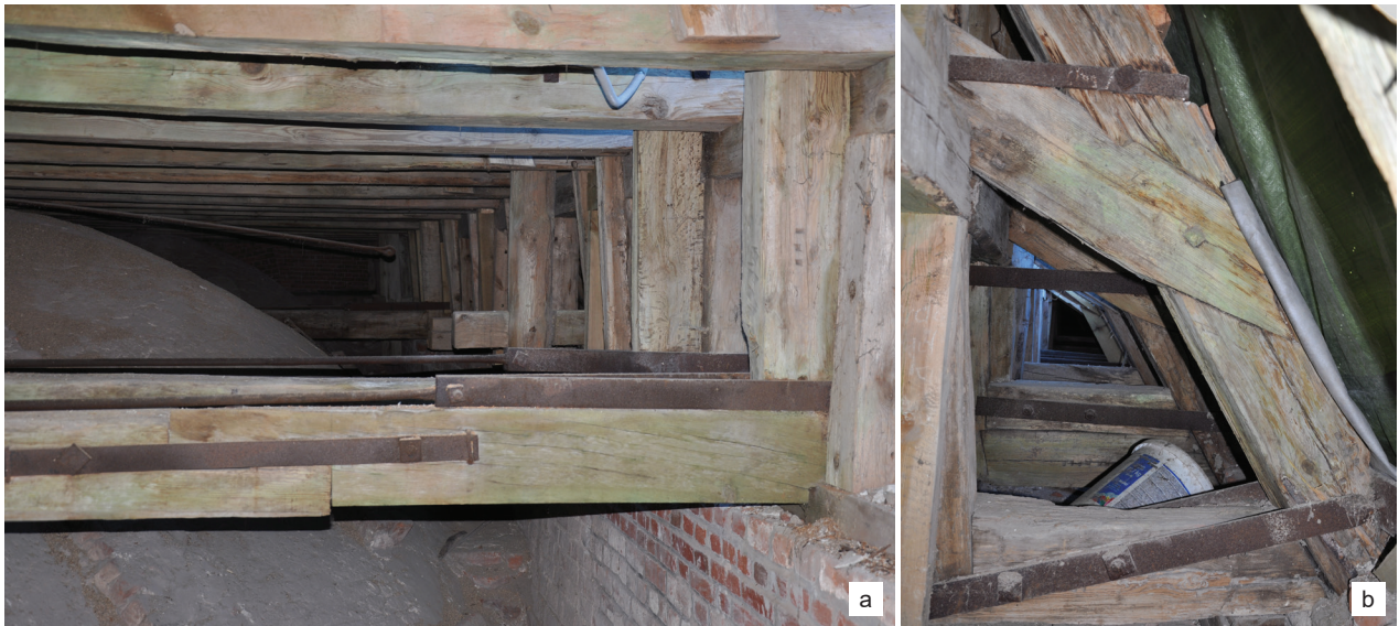
Fig. 9. Kamień Pomorski, cathedral, roof structure above the nave: a) reinforcement of the connection of two parts of the tie beam (principal rafter truss 20) with a flat bar, securing the principal rafter trusses with tensile-resistant anchors (19–20) above the principal rafter truss beam, b) connecting the sole piece with the rafter using two flat bars, joining the (secondary) upper plate with the passing brace and rafter using a flat bar (photo by U. Schaaf, M. Prarat)
