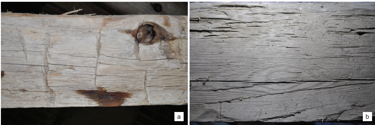
Fig. 4. Kamień Pomorski, cathedral, roof structure above the nave: a) initial processing of wooden building material made with an axe, b) smoothing of pre-processed wooden building material made with an adze (photo by U. Schaaf, M. Prarat)
