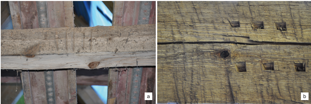
Fig. 3. Kamień Pomorski, cathedral, roof structure above the nave: a) assembly mark in the form of straight lines made with a hand axe, b) assembly mark in the form of rectangular cuts made with a chisel, building material processed from the side of timber framing with a hand saw (photo by U. Schaaf, M. Prarat)
