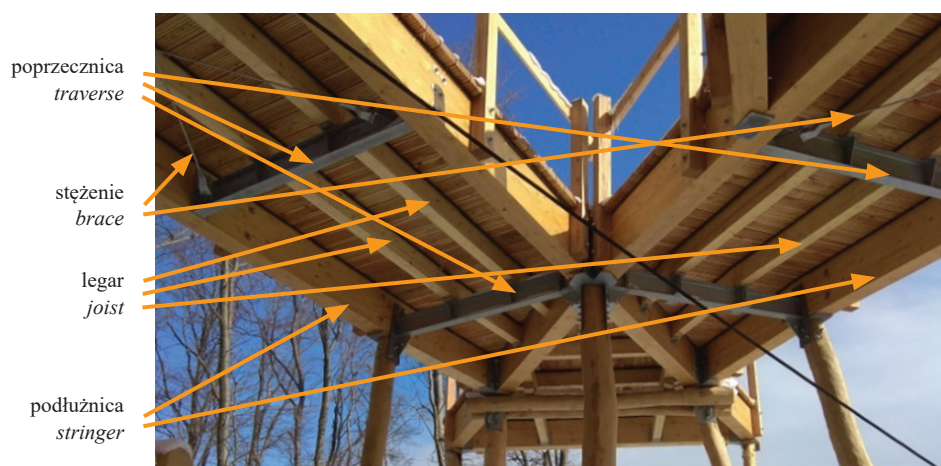
Fig. 11. General view of the construction elements of the ramp of the observation tower in Krynica-Zdrój (photo by S. Czernik)
