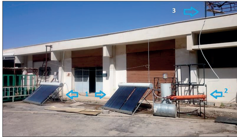
Figure 2. Experimental apparatus: 1 – solar collectors, 2 – heat exchanger, 3 – condenser
