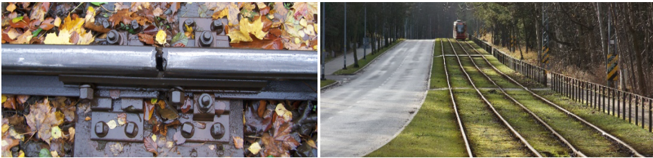
Fig. 4. Examples of critical and very bad technical condition of tram tracks
