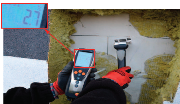
Photo 7. Partial measurement of the mass moisture of the wall substrate in the P1 cut-out – result 2,7%
