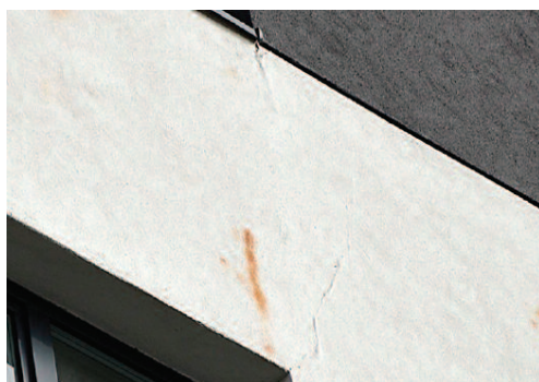
Photo 1. Scratches visible on the surface of the plaster and rust-colored discolorations
