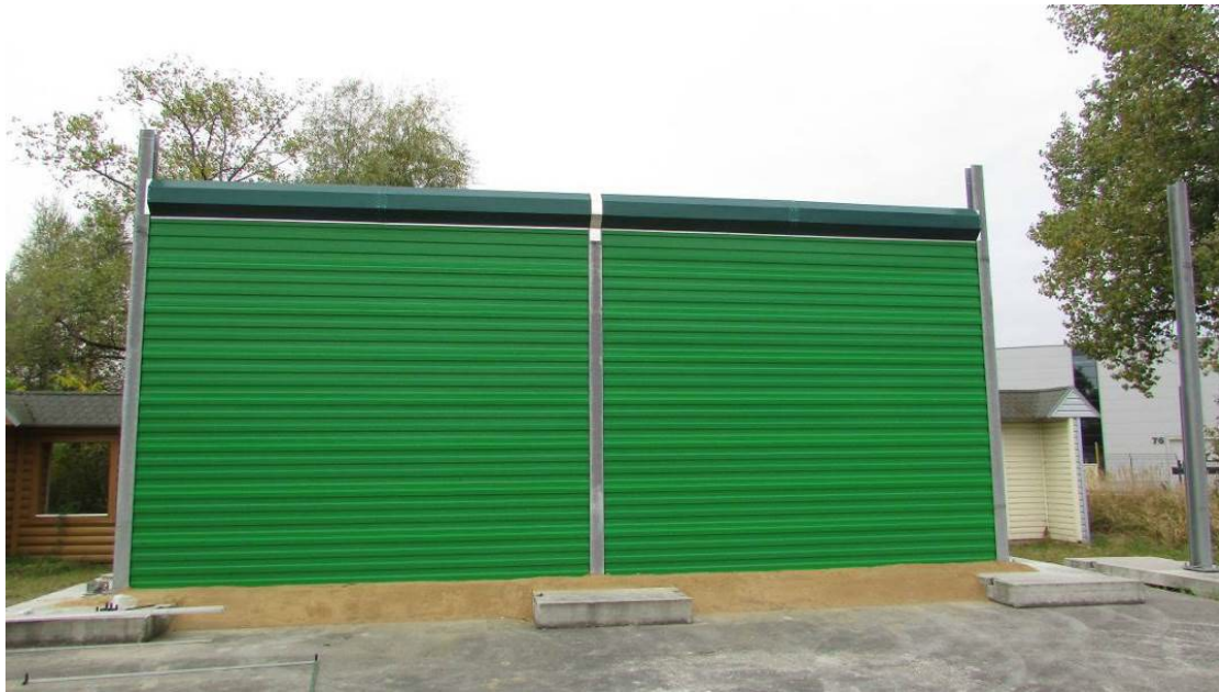
Figure 2. The noise barrier with the added device installed on the top edge.
