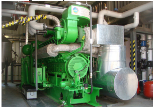
Fig. 1. The GE JENBACHER JMS 316 GS-B.LC Engine Biogas Cogeneration Set operated at the WARTA S.A. Waste Treatment Plant of Czestochowa
