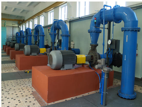
Fig. 1. Pumping station – general view
