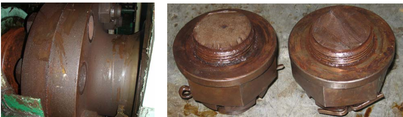
Fig. 8. The view intermediate shaft collar with broken bolts and fractures cross-section of the failed bolts with nuts. [4]
