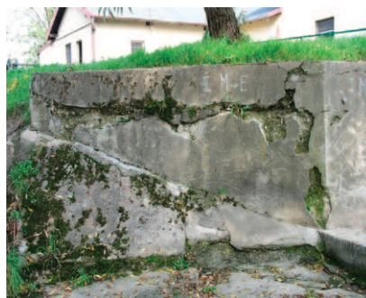
Photo 2. Cracked part of the retaining wall at the fixed weir HP Ławica
