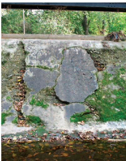
Photo 1. Damaged concrete structure of permanent weir at relief channel HP Ławica
