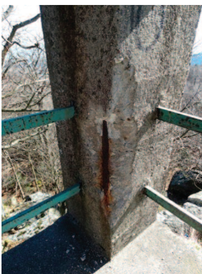
Photo 6. Typical damage to floor slab, beams and columns
