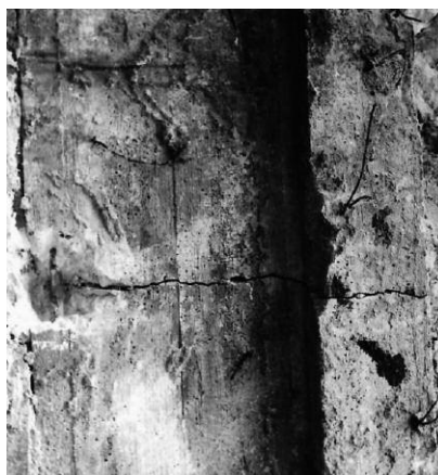
Photo 4. Horizontal cracks in the pole on the Krasinski Street side
