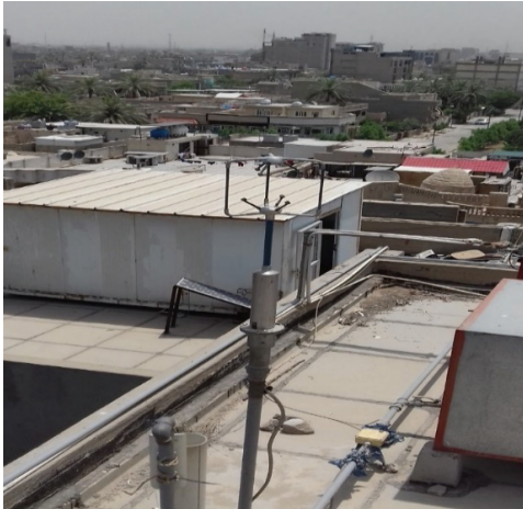
FIGURE 1. Ultrasonic anemometer installed on ASB
