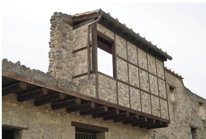
Fig. 36. Herculaneum - an example of a light-weight skeletal wall supported by wooden brackets on the first floor wall. Source: author's photo
