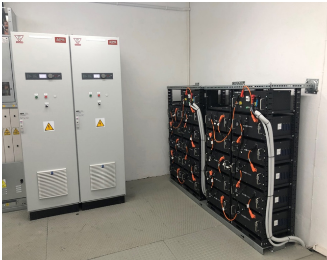
Fig. 6. Twin energy storage systems of APStorage type
