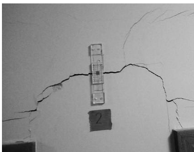
Photo 1. Examples of damage to partition walls as a result of excessive deflection of a floor slab
