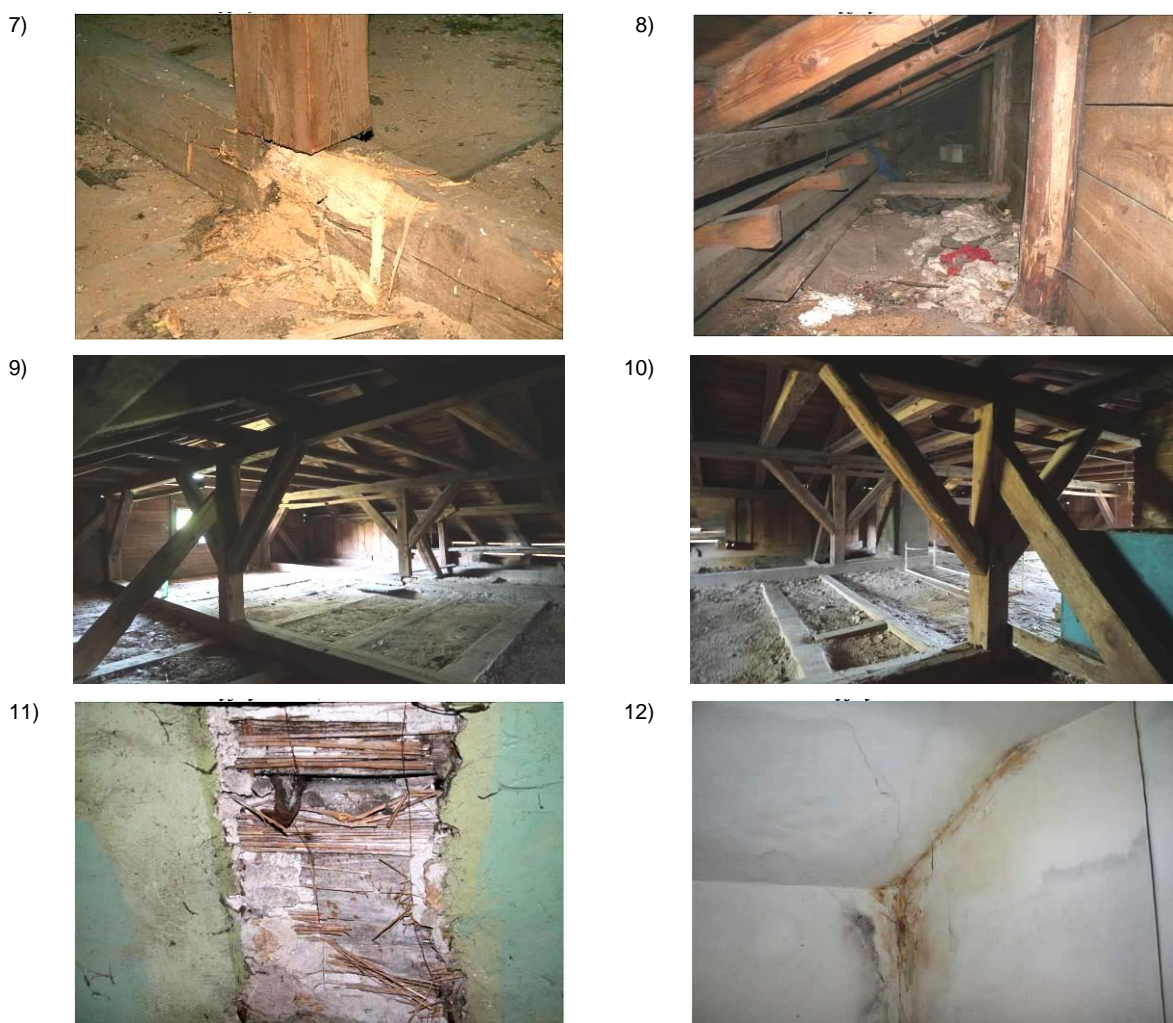
Fig.7-12. Existing condition of the roof structure: 7 – local damage caused by house borer beetles, 8 – eave structure, in satisfactory condition, 9 and 10 – view of rafter-collar tie truss supported by two joist walls over the central part of the manor house, 11 – decay of internal plaster on wooden walls, 12 – dampness of first floor walls. Source: 7, 8,11,12 – Ekspertyza , 2012, 9,10 – original photo 2023
