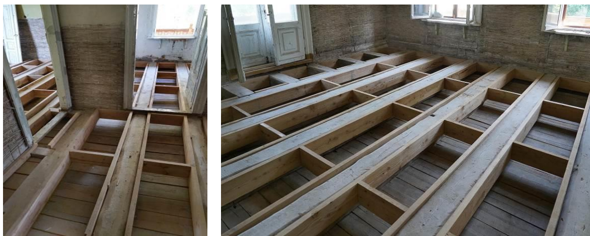
Fig. 27, 28. Conservation renovation of the Rzuców manor house – first floor, reinforcement of wooden ceiling beams. Source: original photo, 2023
