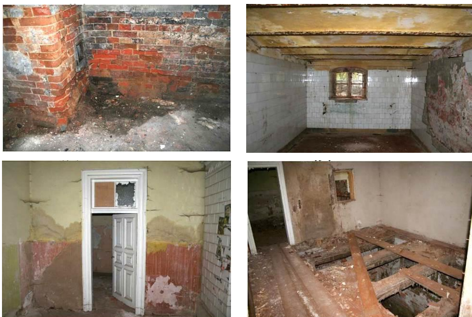
Fig. 3-6. Example of the decay of the load-bearing structure of the manor house – dampness of basement and ground floor walls, and corrosion of segmental vaults at steel beams and deterioration of timber ceilings. Source: Ekspertyza ..2012
