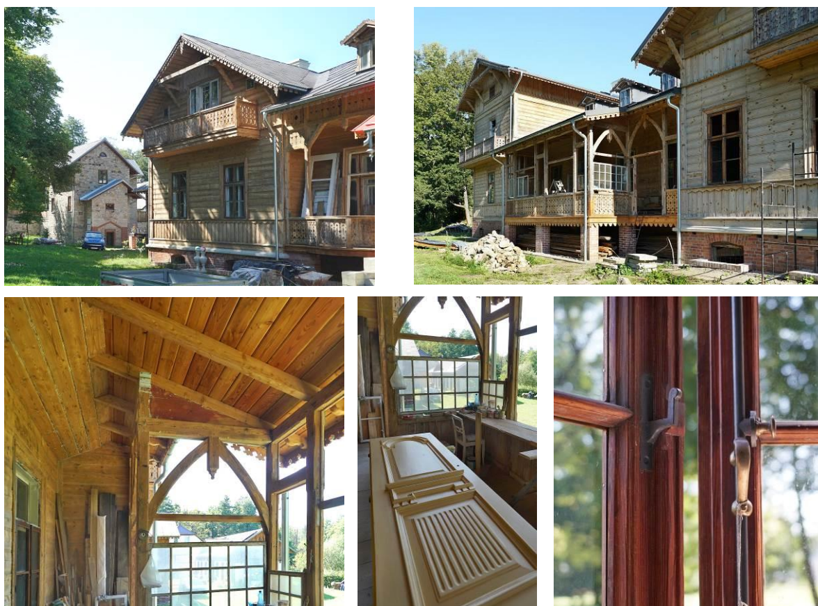
Fig. 44-48. Conservation repairs of the Rzućów Manor House: fragment of the northern facade – in the background a brick building, the so-called 'vicarage' (top left), the northern facade with a veranda, the so-called 'winter garden' (top), fragment of the veranda structure, conservation of the inner door leaf – with restoration of the original colouring, window fragment after cleaning. Source: original photo 2023
