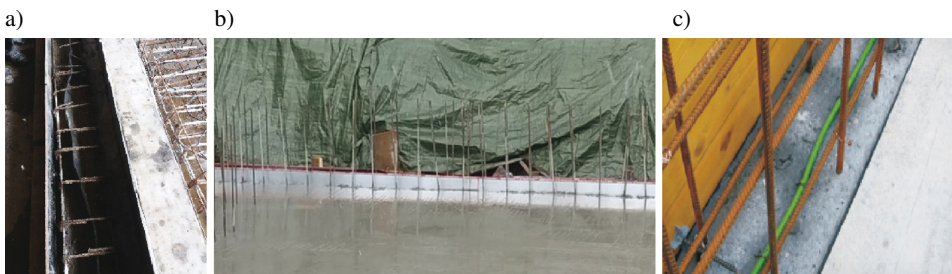
Fig. 3. Systems based on: a) “rubber” joints, b) “metal sheets”, c) injection hoses (authors’ archives)
