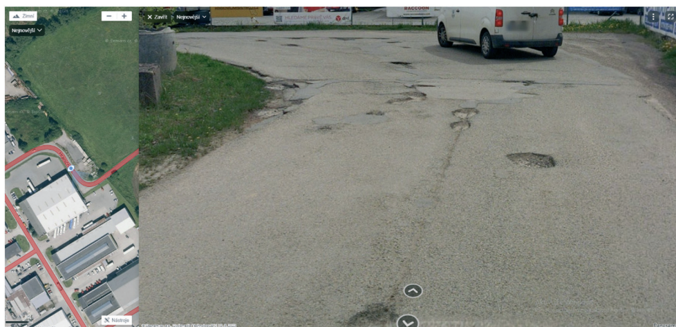
Fig. 4. Wrong road condition [10]
