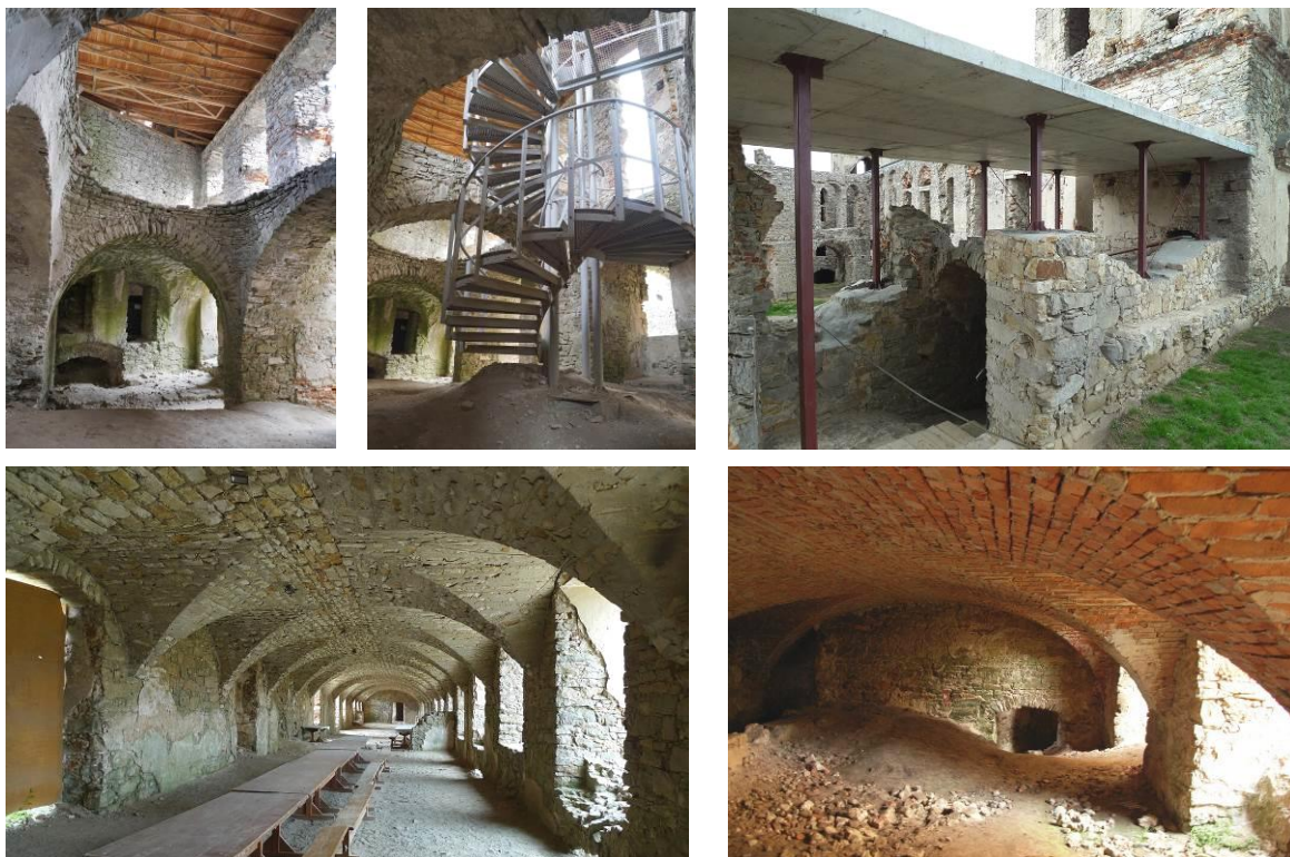
Fig. 77-81 Krzyżtopór Castle - despite the successful reconstruction of some of the degraded vaults according to the reconstruction project in the 1970s-80s, unfortunately in 2010-2013 it was already limited to the introduction of strange flat modern roofs and stairs and reinforced concrete roofs, foreign in style and material (top) - surprisingly agreed with the conservation authorities! Source: photos by author, 2012
