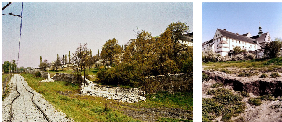
Fig. 3 Wieliczka, destroyed railway tracks and the wall of the Franciscan-Reformed monastery in the centre of the subsidence basin formed after the catastrophic water leakage into the Mina crosscut in 1992 (photo: J. Przybyło)
