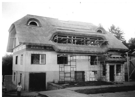
FIGURE 3. Ecological thermal modernization of a building from the end of 1970's consisting in construction of a superstructure and covering the house with a step roof. An attempt of reference to tradition – a thatched gable roof with jerkin head. Some reservations can be expressed about the building enormity, resulting from the high cellar, differing from that historically developed – Minkowice, July 2008 (photo by Autor)
