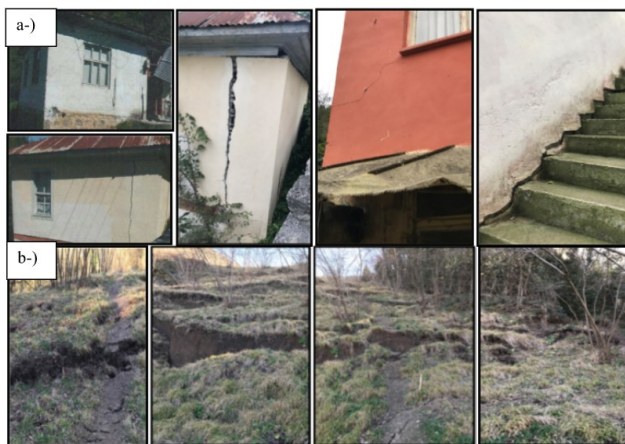
Figure 2. a) The mass movement-induced damage of the constructions in the study area. b) The surface cracks as a result of mass movements in the study area.
