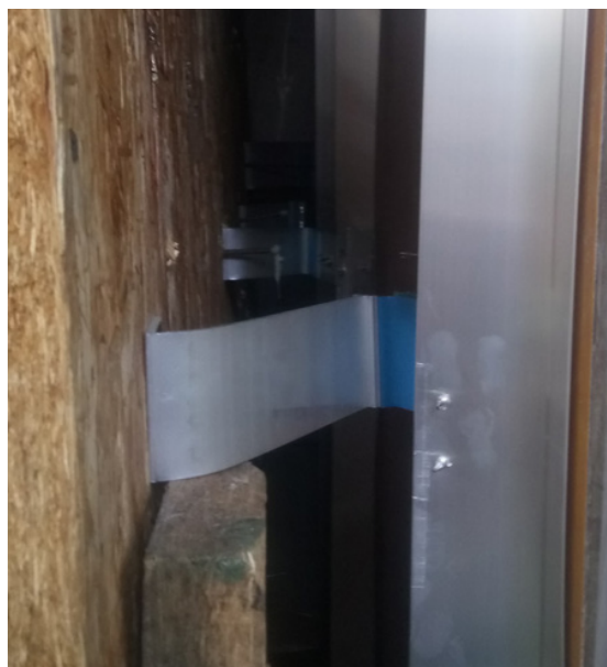
Photo 1. Deformation of the brackets in the rainscreen system under horizontal loading – wind pressure
