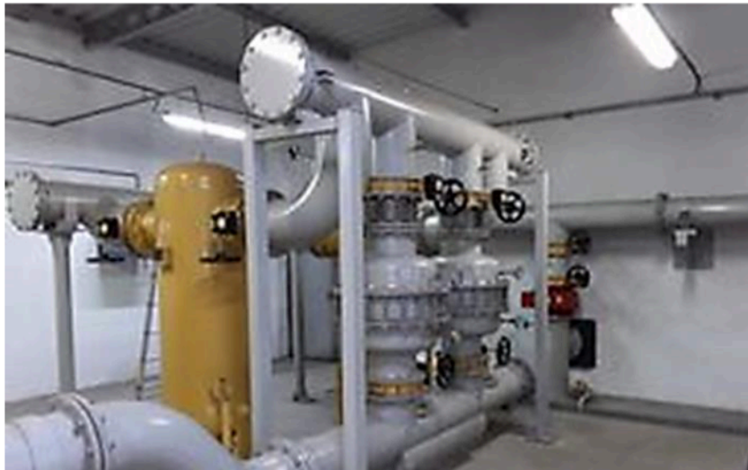
Fig. 2. Equipment of the methane drainage station at the methane inlet
