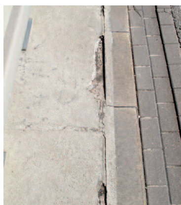
Photo 3. Losses of waterproof pavement membrane in the curb zone caused by degradation of the concrete
