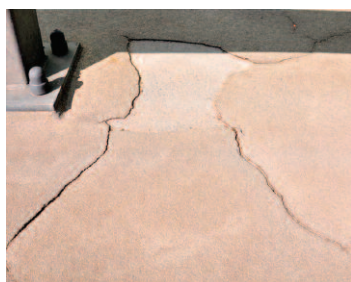
Photo 1. View of the waterproof pavement membrane based on epoxy-polyurethane, cracked and detached from the concrete base
