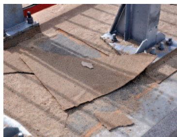
Photo 2. View of the waterproof pavement membrane based on MMA (methyl methacrylate); detachment occurred between the primer and base layers
