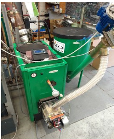
Fig. 3. 20 kW boiler with a pellet furnace equipped with rotary combustion chamber, installed in a full scale experimental heat station; thermocouple above the furnace
