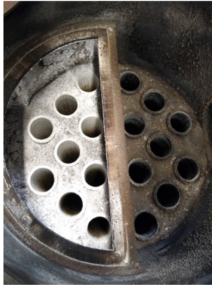
Fig. 5. Deposits in the boiler after firing a mixture of coffee husk pellets and wood pellets at a weight ratio of 70:30
