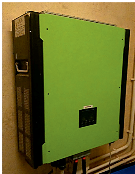
Fig. 3. A photograph of the frequency converter (photo P. Świsłowski)
