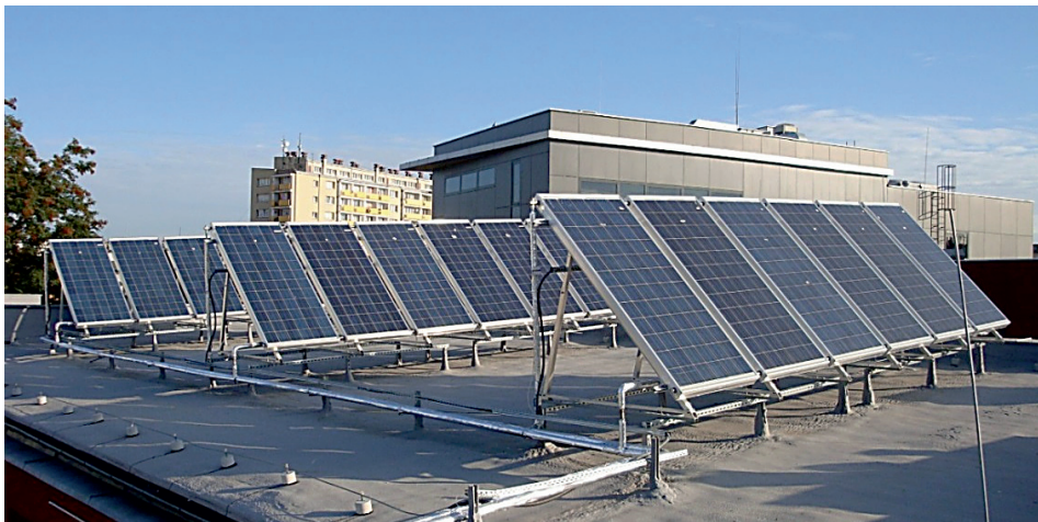
Fig. 2. A photograph of the PV system installed on the roof of University of Opole building (photo P. Świsłowski)
