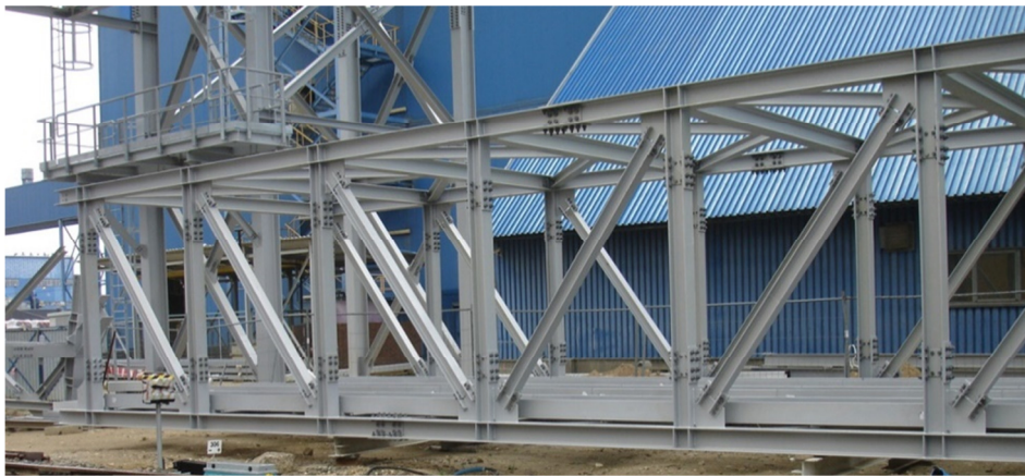
Fig. 1. Disassembled span of the conveyor structure [photo: A. Biegus]
