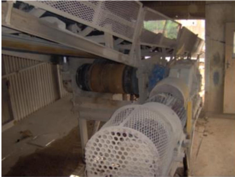
Fig. 1. Conveyor belt drive
