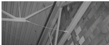
Fig. 4. Overextended strut due to improper prestress [29].
