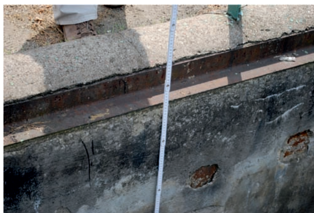
Rysunek 3 Widok ubytków betonu w ścianie zbiornika Figure 3 View cavities in the walls of the tank
