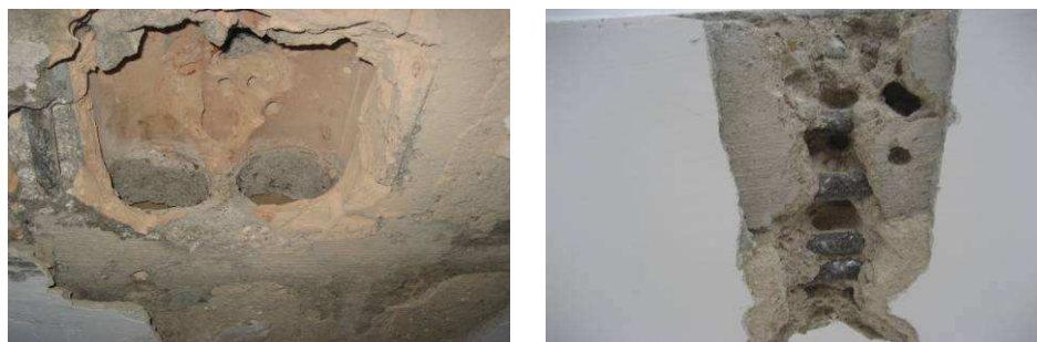
Fig. 6. Test openings in the ceiling above the basement: the floor slab (left) and the main beam (right)
