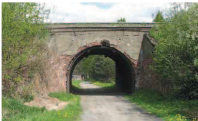
Rys. 1. Ceglany wiadukt łukowy pod torem nr 1 [9] Fig. 1. Brick arch viaduct under railway track no. 1 [9]
