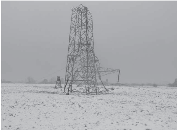
Fig. 6. Damaged poles of a high voltage power supply Szczecin [10]
