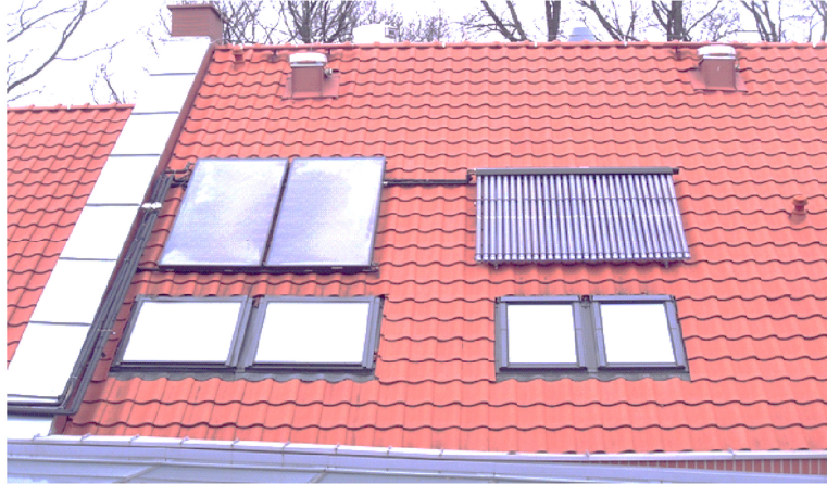
Fig. 1. Location of flat-plate collectors (on the left) and evacuated tube (on the right) on the roof of the building Institute of Construction in Olsztyn ( own study )
