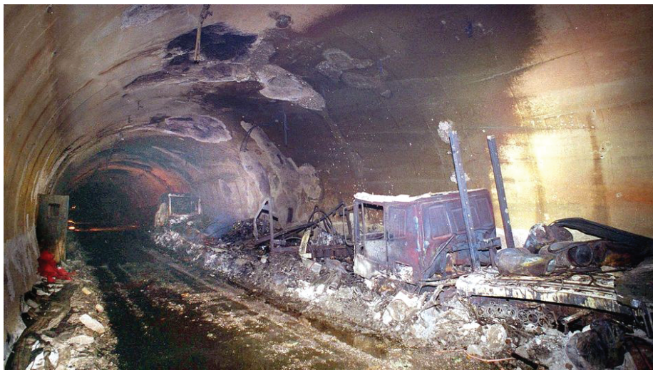
Fig. 1. Result of the fire in the Mont Blanc road tunnel [2]
