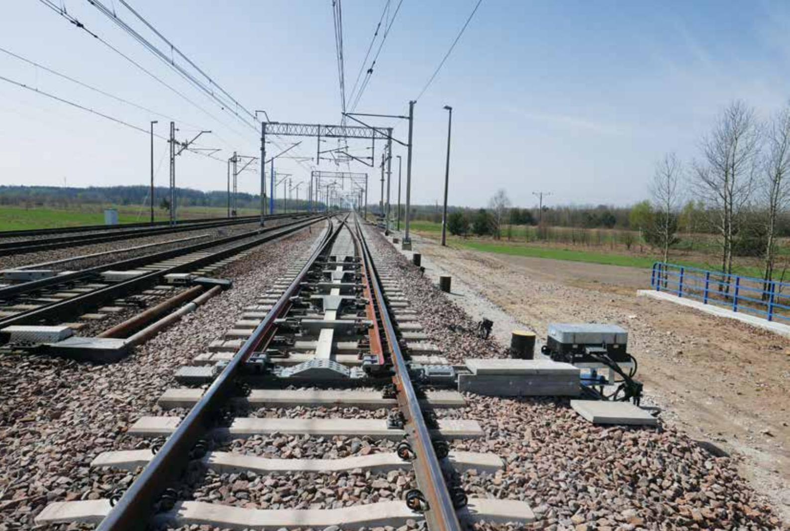
Fig. 1. Turnout R1200, 1:18.5 switch panel. Photo shows the MOT (first actuator), actuators #2, #3 and #4 and blade struts between actuators. HPU is installed on the right side of the track Source: own archive.
