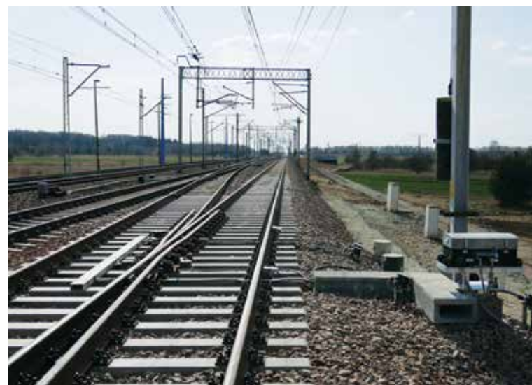
Fig. 2. Turnout R1200, 1:18.5 crossing. Actuators, trailing controller, ARES turnout heating separation transformers, JVA terminal boxes and HPU Source: own archive.
