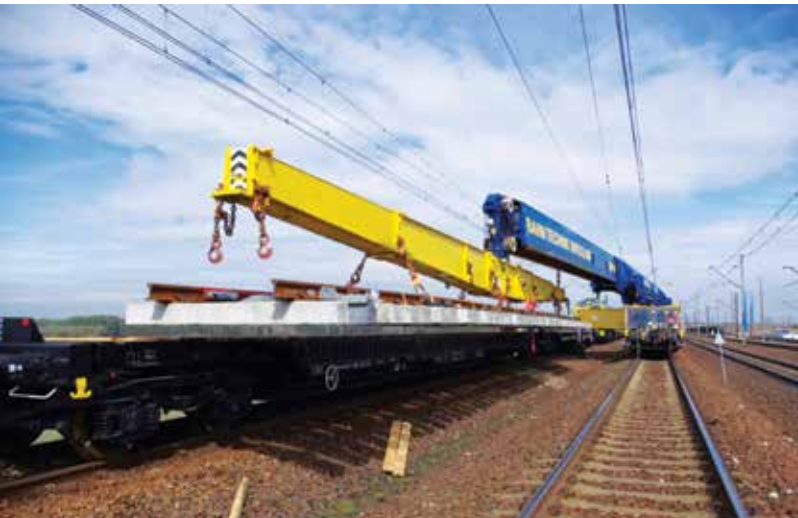
Fig. 5. Special railway crane Gottwald GS 150.14TR during turnout installation at the Psary Station Source: own archive.
