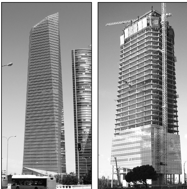
Figure 14: Torre de Cristal, Madrid: a view – the form and the steel and concrete structure under construction source: J. Pietrzak and upload.wikimedia.org/wikipedia/commons/a/a1/Torre_de_Cristal_%28Madrid%29_03a.jpg
