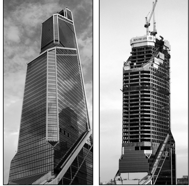
Figure 12. Mercury City Tower, Moscow: a view – the form and the reinforced concrete under construction. source: www.skyscraperpage.com/showthread.php?t=351203&page=178 and www.schoeck.com/en/media-relations/reaching-the-sky-europe-s-tallest-building-incorporates-schoeck-thermal-break-technology-344?filter-active=1
