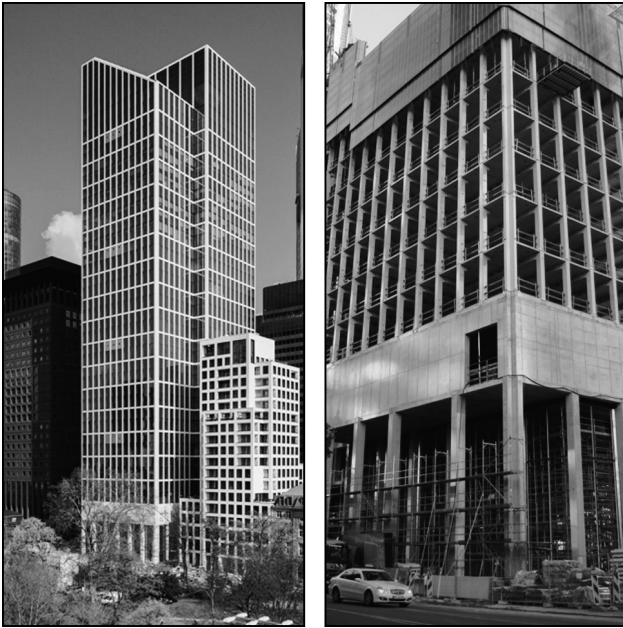
Figure 7. Taunus Turm, Frankfurt: a view – the form and the prefabricated concrete structure under construction. source: www.hofmannnaturstein.com/files/taunusturm-frankfurt_03_neu.jpg and http://www.skyscrapercity.com/showthread.php?t=521026&page=22
