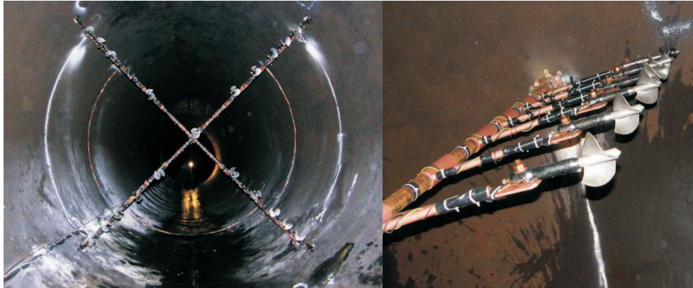
Figure 9: Current-meters and the Gibson method impulse tubes in the penstock of Zur hydropower plant.
