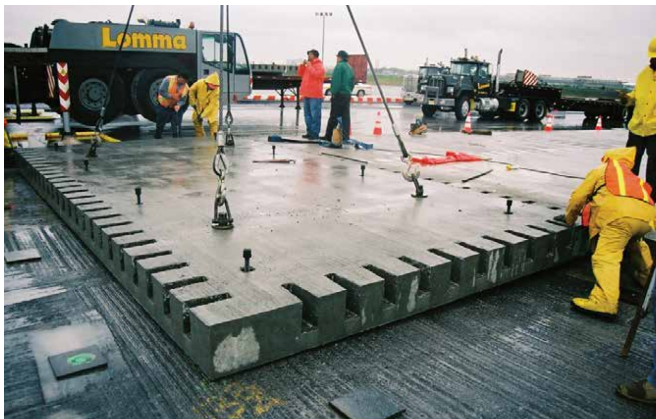
Fig. 1. Prefabricated PCP concrete slab used at La Guardia International airport in New York [2]
