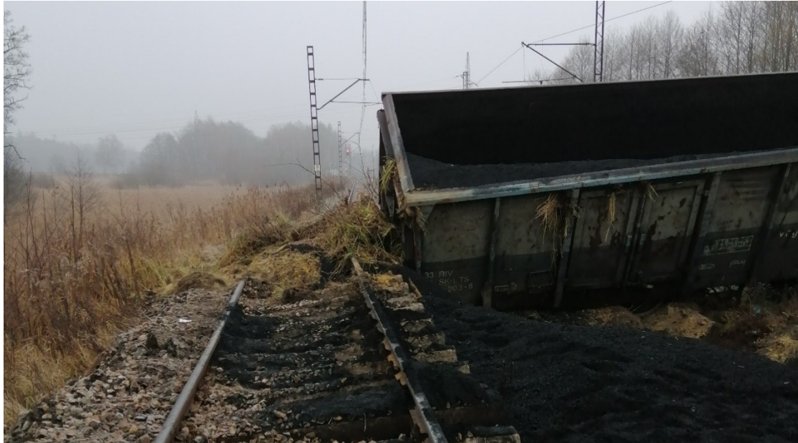
Figure 5. On-site inspection of B09 accident. The second derailed wagon.
