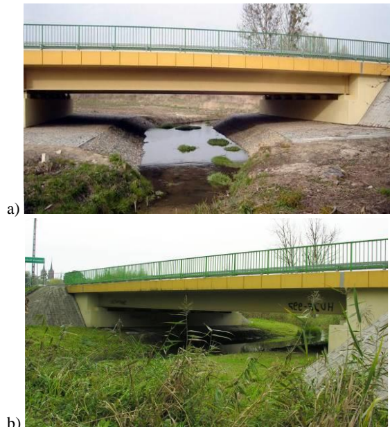
Figure 5. The bridge over the Lopa River in Lopiennik; transition for medium-sized animals a) in 2007 b) in 2009
