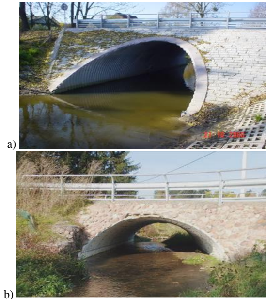
Figure 4. River culverts designed in accordance to old and new standards a) built in 2006 b) constructed in 2013
