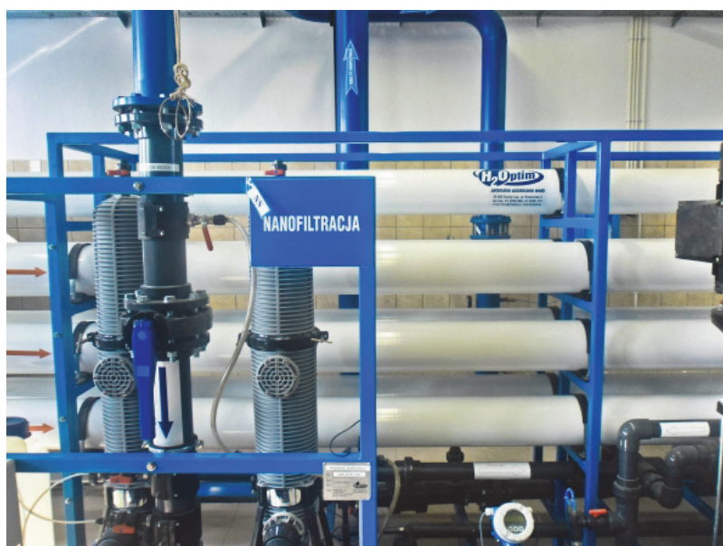
Fig. 4. The photograph of installation for water treatment operated at WTP Zawada n/Dębica (ABT 2013)
