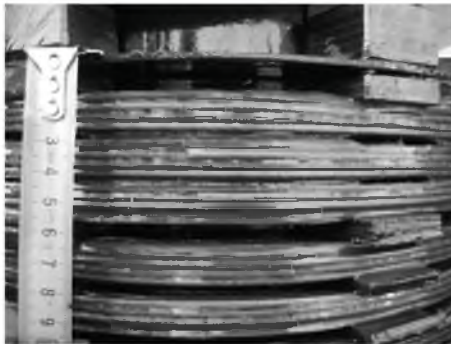
Fig. 7. Transformer winding with deformation D3 – top two discs lowered to minimum
