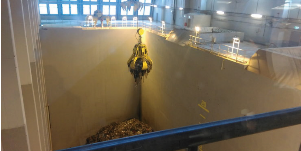
Fig. 4. Waste bunker with a visible industrial crane
