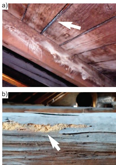
Photo. 4. Selected construction problems: a) cracks visible in solid wooden boards and severe moisture in elements; b) traces of insect activity
