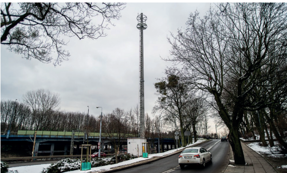
Fig. 4. Telecommunications mast in PKM traffic control system [own study]
