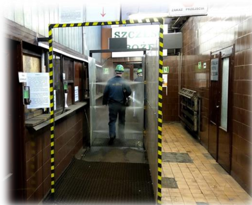
Fig. 8. A prototype of the UMID universal disinfecting installation in Budryk mine, made by Elektron s.c. [18]
