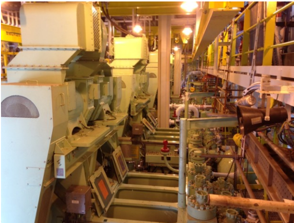
Fig. 5. A view of the mud pumps section of a drilling rig's power plant
